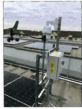
10 E40 ALSOENERGY WEATHER STATION
