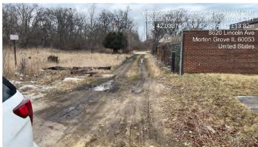
Photo of Unpermitted Cut-through
