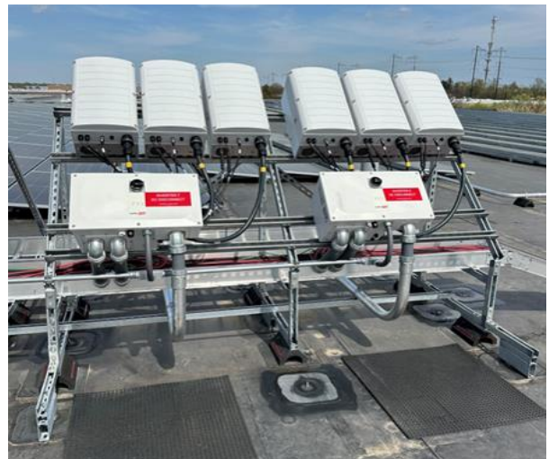
Example of an unscreened Inverter Rack (with two inverters)
